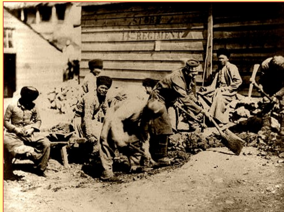
Fenton, Roger (1819-1869) (photographer) (1855) Tartar labourers repairing road in Balaklava, British regiment, Crimean War Library of Congress Prints and Photographs Division Washington, D.C. 20540 USA lcloc.gov/2001697109 cdn.loc.gov/service/pnp/cph/3a40000/3a47000/3a47600/3a47689r.jpg
