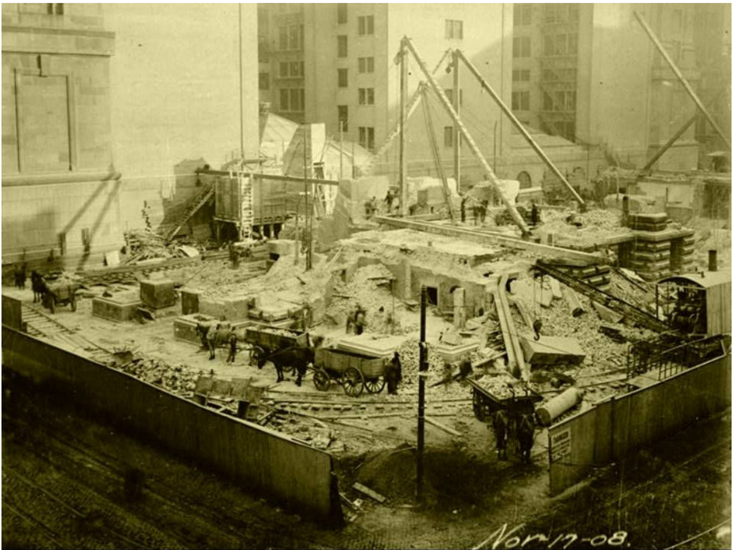
21. Demolition down to ground floor, showing skylights and upper stories of new county building, Nov. 17. 1908 - Chicago City Hall, 121 North LaSalle Street, Chicago, Cook County, IL
