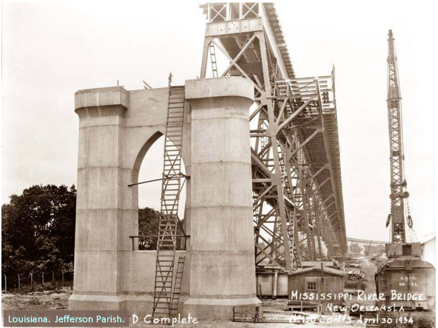
Louisiana. Jefferson Parish. D Complete Contract number 3 showing main bridge Pier D complete. Unknown (original photographer) (1934 April 30). Photo 139 of 213. HAER LA-17/ Marcus Lamkin (creator/ photographer) (2005)
