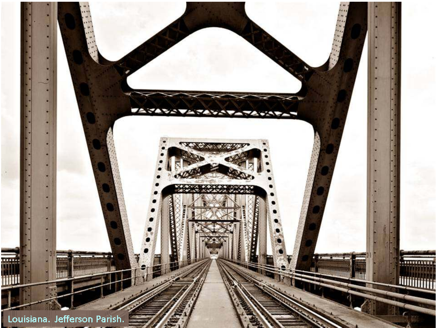
Huey P. Long Bridge, Spanning Mississippi River approximately midway between nine & twelve mile points upstream from & west of New Orleans, Jefferson, Jefferson Parish (LA). HAER LA 17/ Marcus Lamkin (creator/ photographer) (2005).
