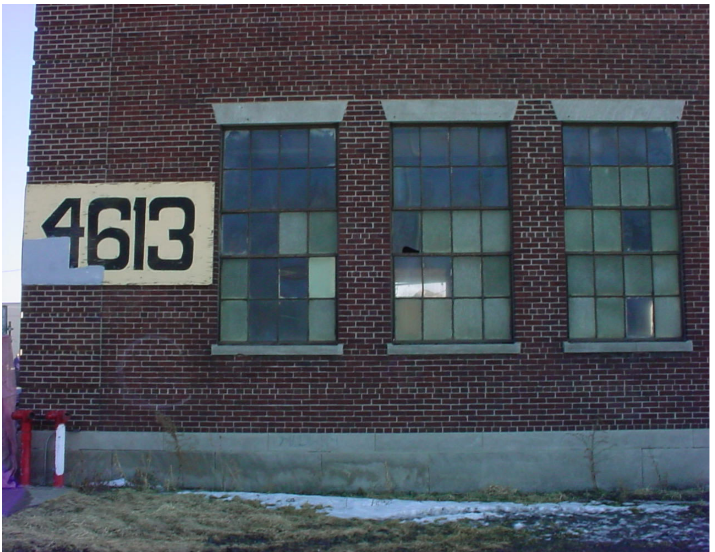
2005-02-04. Western Avenue 4500-4600S. Industrial conversion to retail. Shoppers Paradise (Shoppers Paradise etc. to Home Depot and empty lots.) Demolition days.
