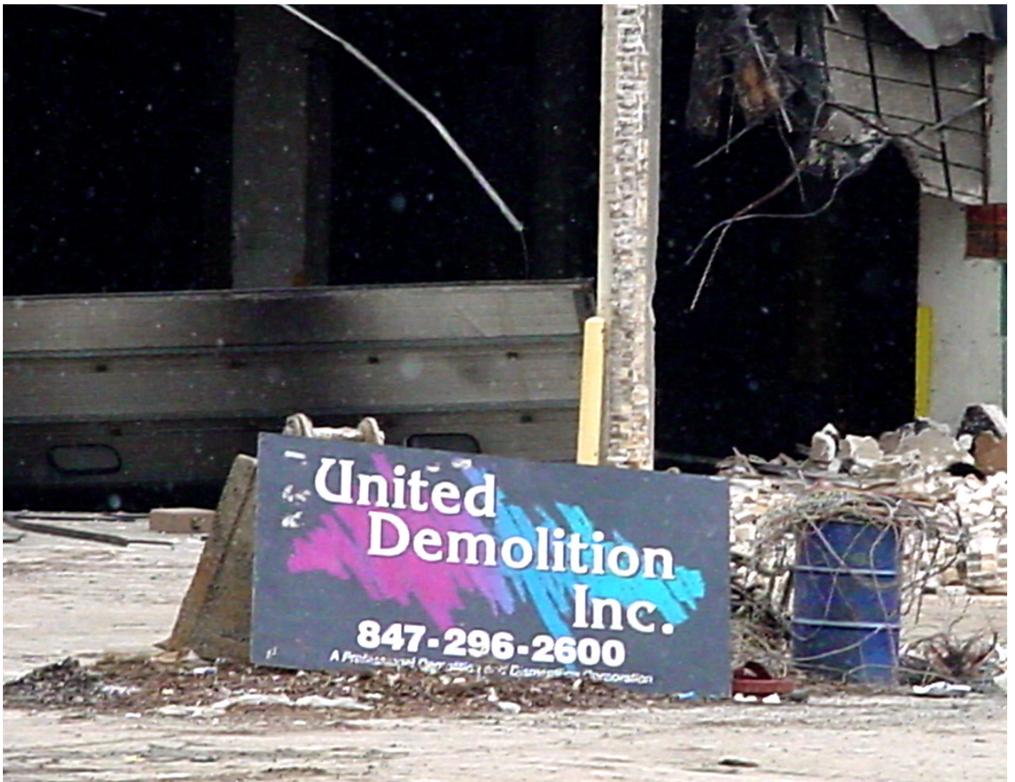
2005-02-24. North Avenue 4630W. Conversion of industrial to retail. (Giant productive Helene Curtis complex to Walmart. Demolition Days.
