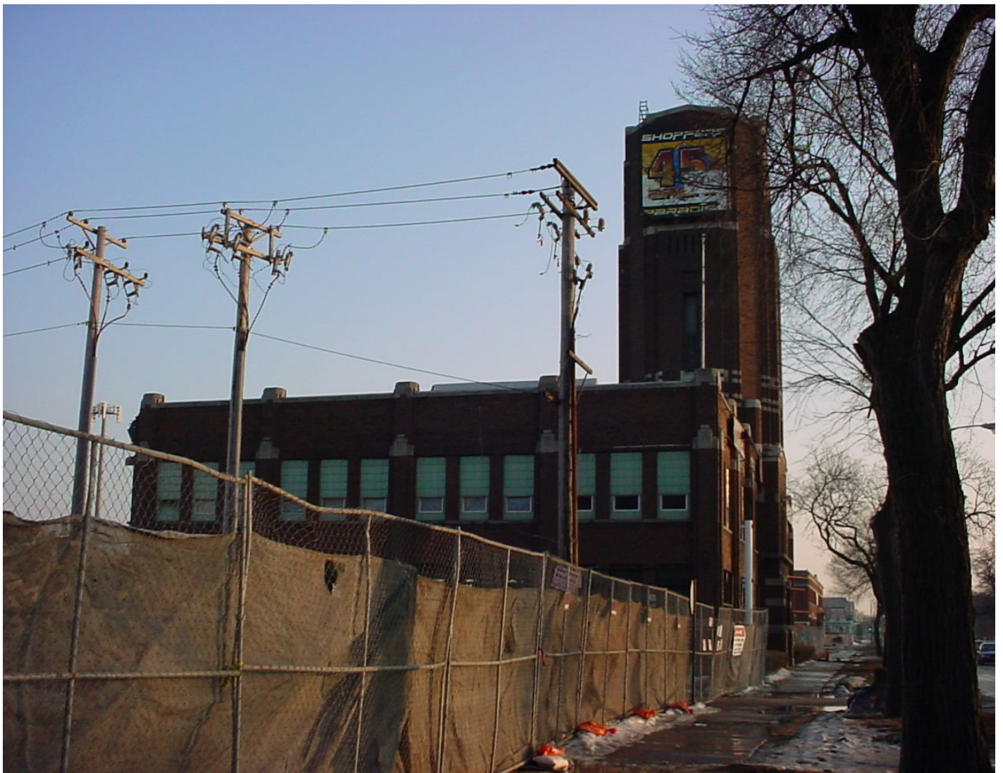
2005-02-04. Western Avenue 4500-4600S. Industrial conversion to retail. Shoppers Paradise (Shoppers Paradise etc. to Home Depot and empty lots.) Demolition days.
