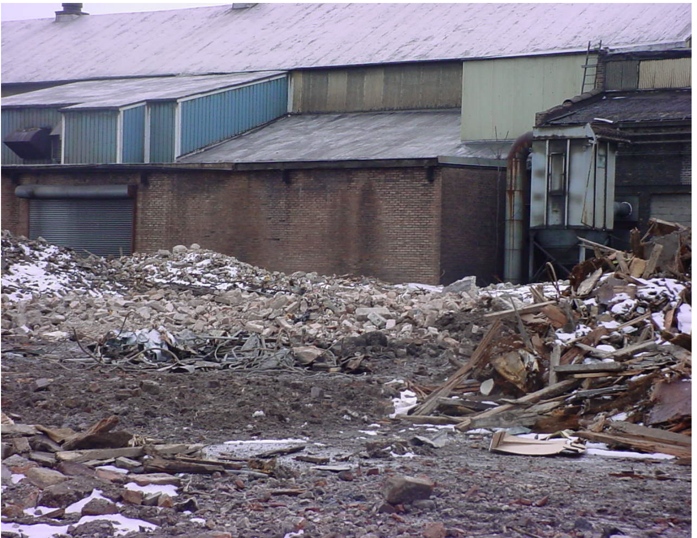
2005-03-04. Taylor Street 2525W Conversion of industrial to residential planned. Francis Nygren Foundry. Demolition Day.
