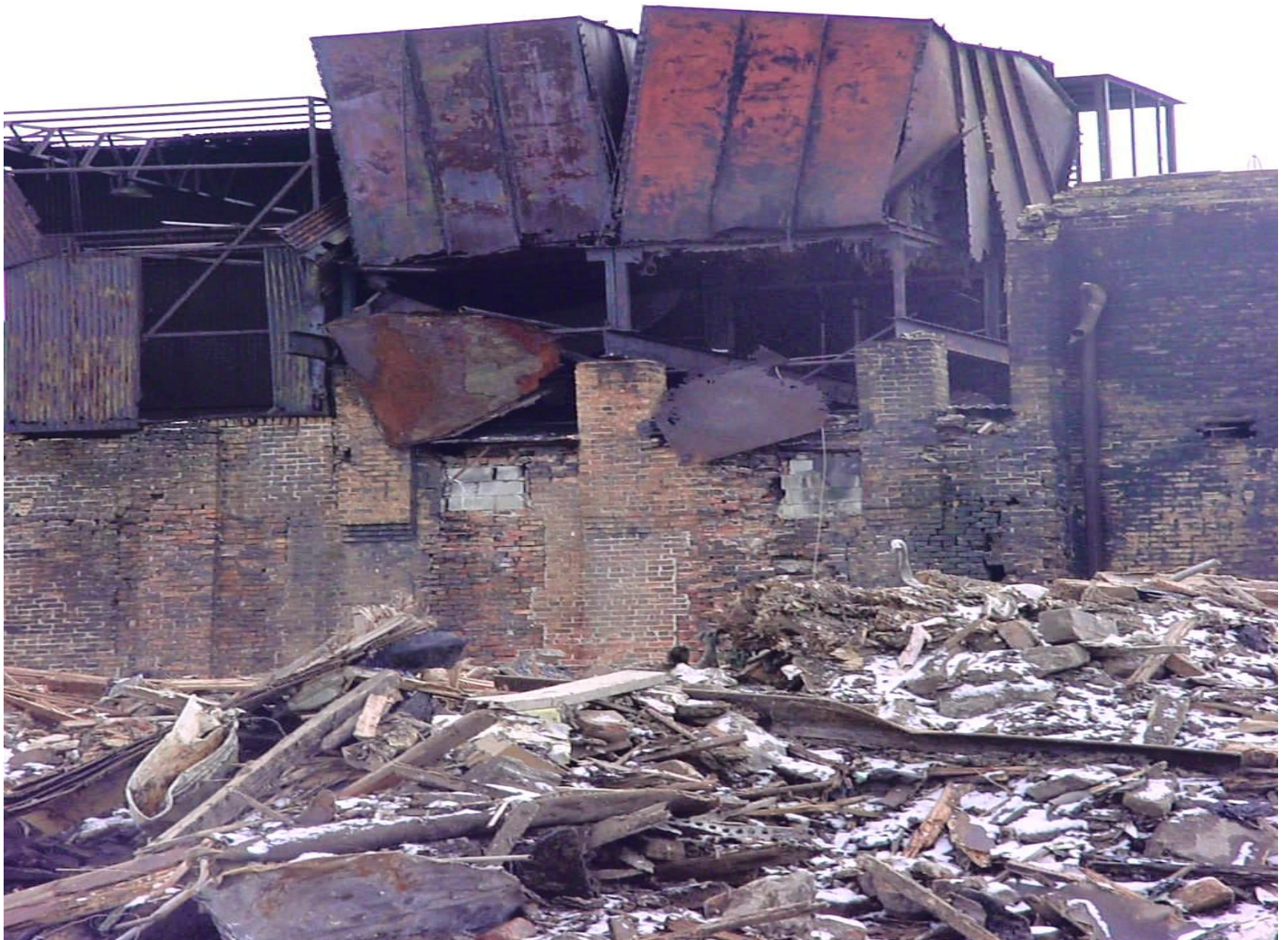
2005-03-04. Taylor Street 2525W Conversion of industrial to residential planned. Francis Nygren Foundry. Demolition Day. .
