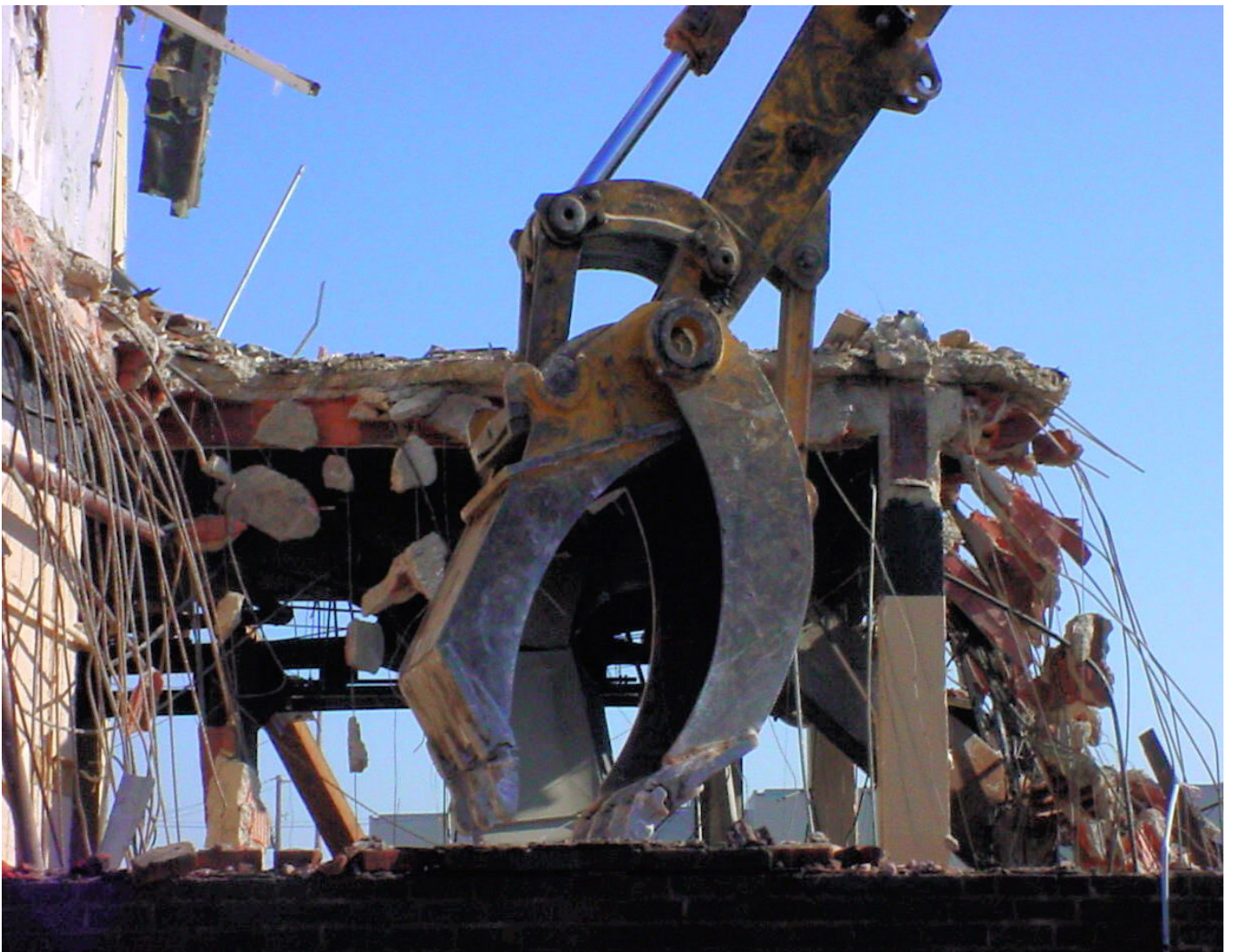
2005-02-04. Western Avenue 4500-4600S. Industrial conversion to retail. Shoppers Paradise (Shoppers Paradise etc. to Home Depot and empty lots.) Demolition days.
