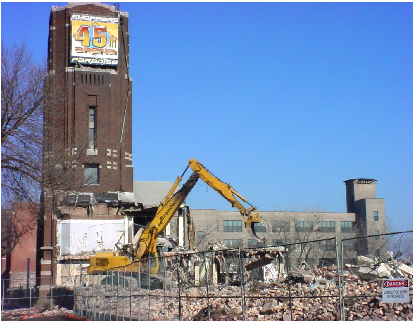
2005-02-04. Western Avenue 4500-4600S. Industrial conversion to retail. Shoppers Paradise (Shoppers Paradise etc. to Home Depot and empty lots.) Demolition days.
