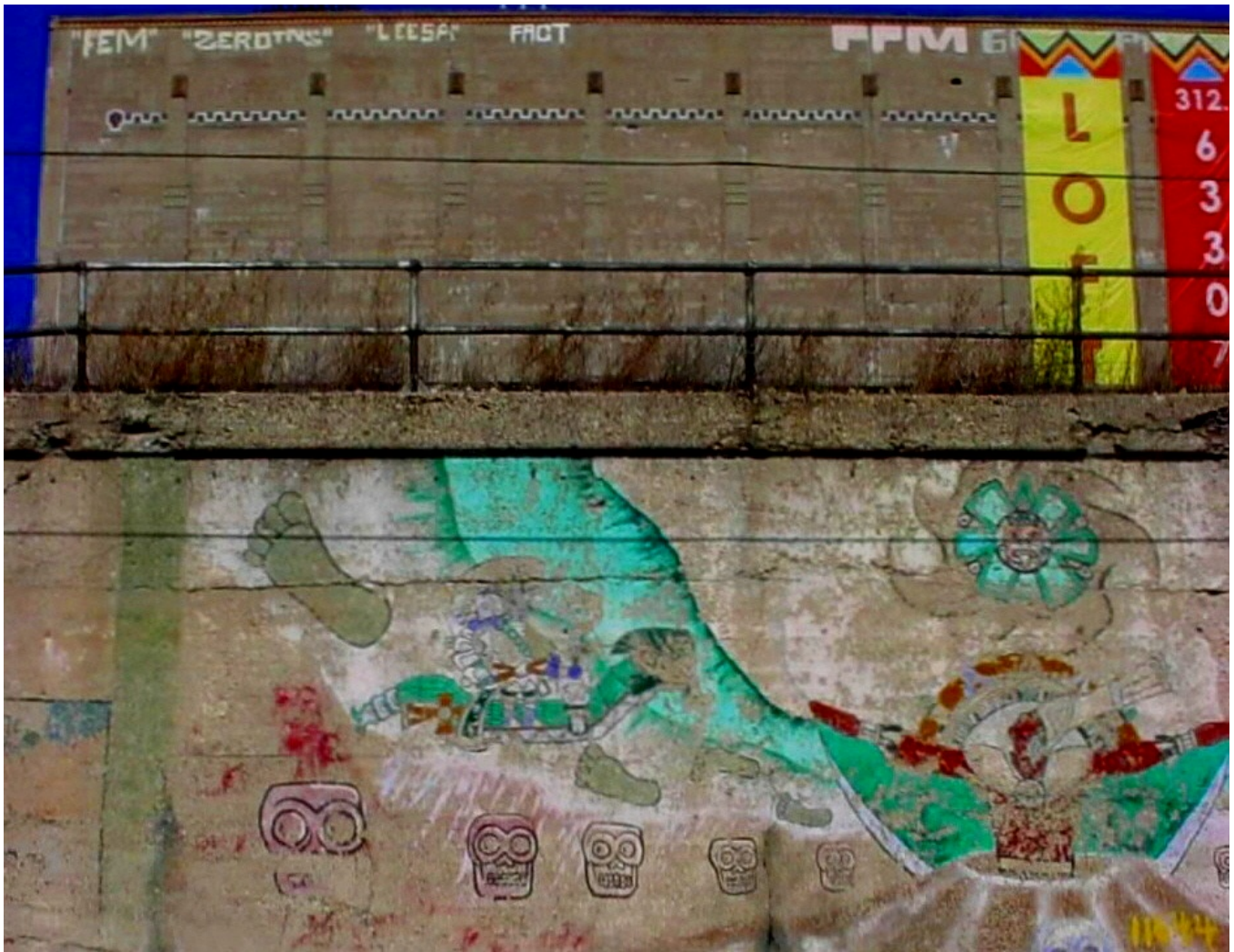
Produce Terminal (south façade, behind elevated railroad tracks) Blue Island 1360S, Chicago, Illinois.
