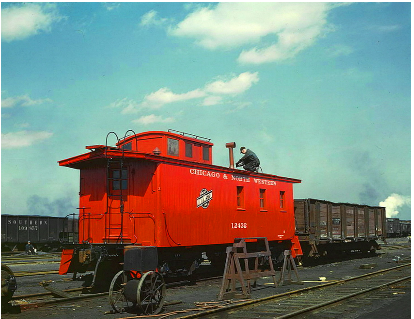
Delano, Jack (1914-) (photographer). C & NW RR, putting the finishing touches on a rebuilt caboose at the rip tracks at Proviso yard, Chicago, Ill.
