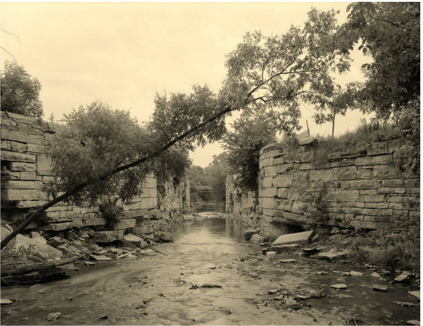
Gooding, William. I&M Canal Lock #2, located about one mile south of Lock #1, in Lockport. Historic American Engineering Record. HAER ILL,99-LOCK,2-6. Lockport Historic District, Illinois & Michigan Canal, Lockport, Will County, IL
