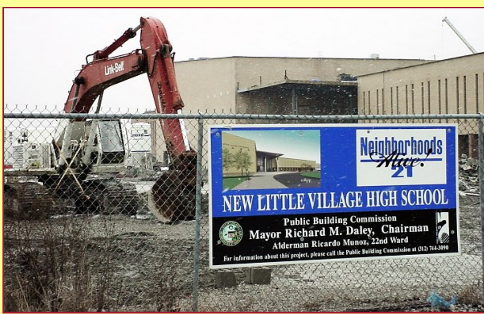
New Little Village High School under construction 35th Street & Kostner 4400W 3500S, Chicago, Illinois (2005 February 28)
