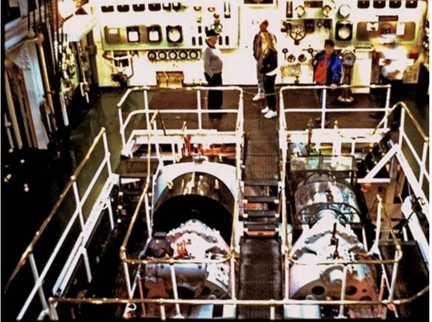
Boiler room of a Great Lakes iron ore carrier.
